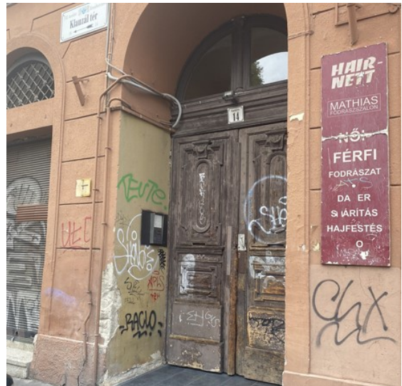
Figure 5. Graffiti on a building and plaster falling off. (Source: the author, 2022)
